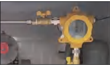
Air conditioning water cooling system
